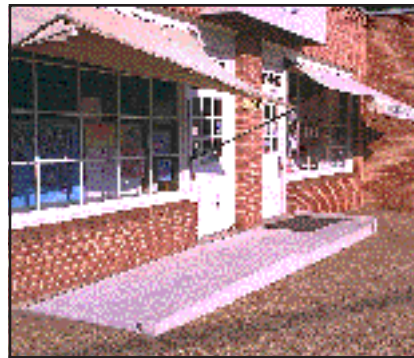
The awning and awning support over the walk to the entrance is too close to the ground and is a barrier to people who are blind or visually impaired.
